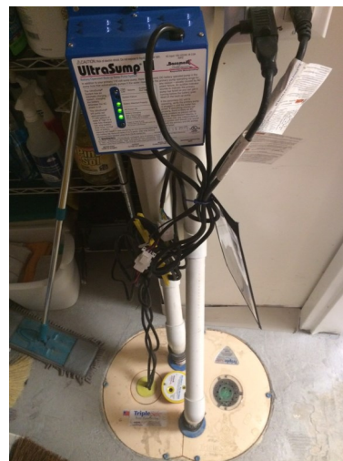
One of the two sump pumps that's been installed.
